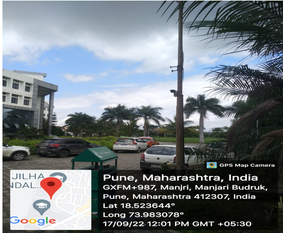
CCTV camera at College Entrance
